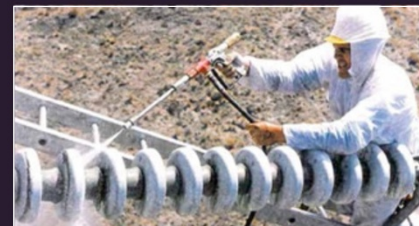
Ash is cleaned from a 220 KV strain insulator string using pressurised water following the 1995 Ruapehu eruption, New Zealand (Transpower New Zealand)
