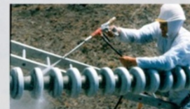
Ash is cleaned from a 110 kV horizontal insulator string using pressurised water following the 1995 Ruapehu eruption, New Zealand. (Transpower New Zealand)
