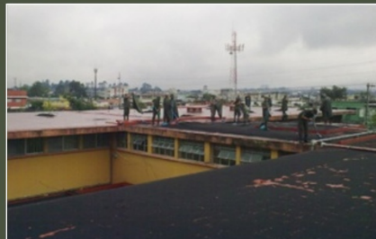
An eruption of Pacaya volcano in 2010 deposited ~20 mm of coarse basaltic ash on Guatemala City. This photo shows cleanup of ash from the roof of a major public hospital. Ash entered gutters and drains, causing flooding. Some abrasion damage to the paint coating on the roof occurred.
