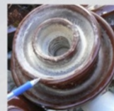
The underside of a 33kV insulator coated in ash, which led to flashover, following ashfalls during the 2008 Chaiten eruption, Chile
