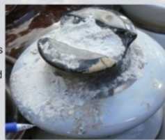
Ashfall covers a 33kV insulator following the May 2008 Chaiten eruption, Chile
