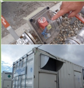
Adaptations to protect GenSet equipment in Bariloche, Argentina, from repeated airborne ash exposure following 2011-2012 eruption of Cordón Caulle volcano, Chile. Top: sealed fuel valve. Bottom: hood to protect air intake.
