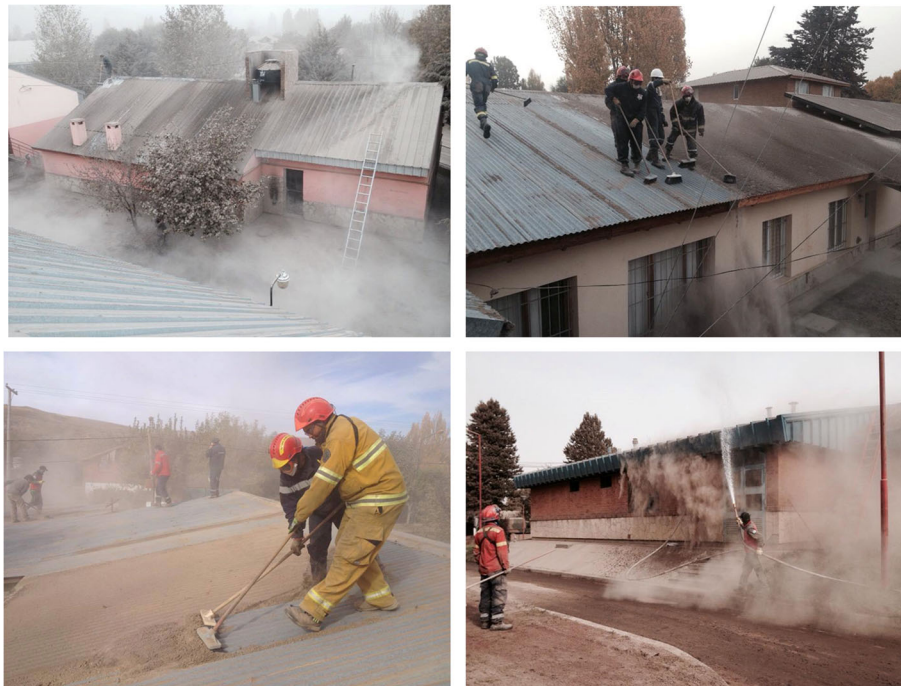
Fig. 7 Cleaning tephra from roofs in Junín de Los Andes (photos courtesy of Junín de Los Andes Bomberos, Date: April 2015)
